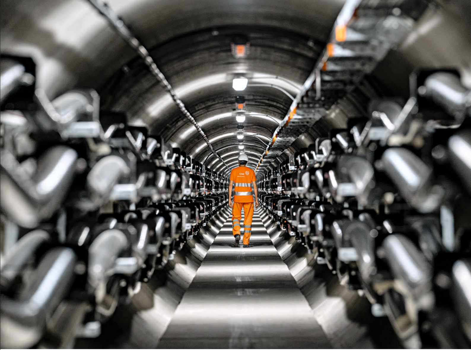
Cable tunnel between La Bâtiaz and Le Verney in the Martigny area (VS)
