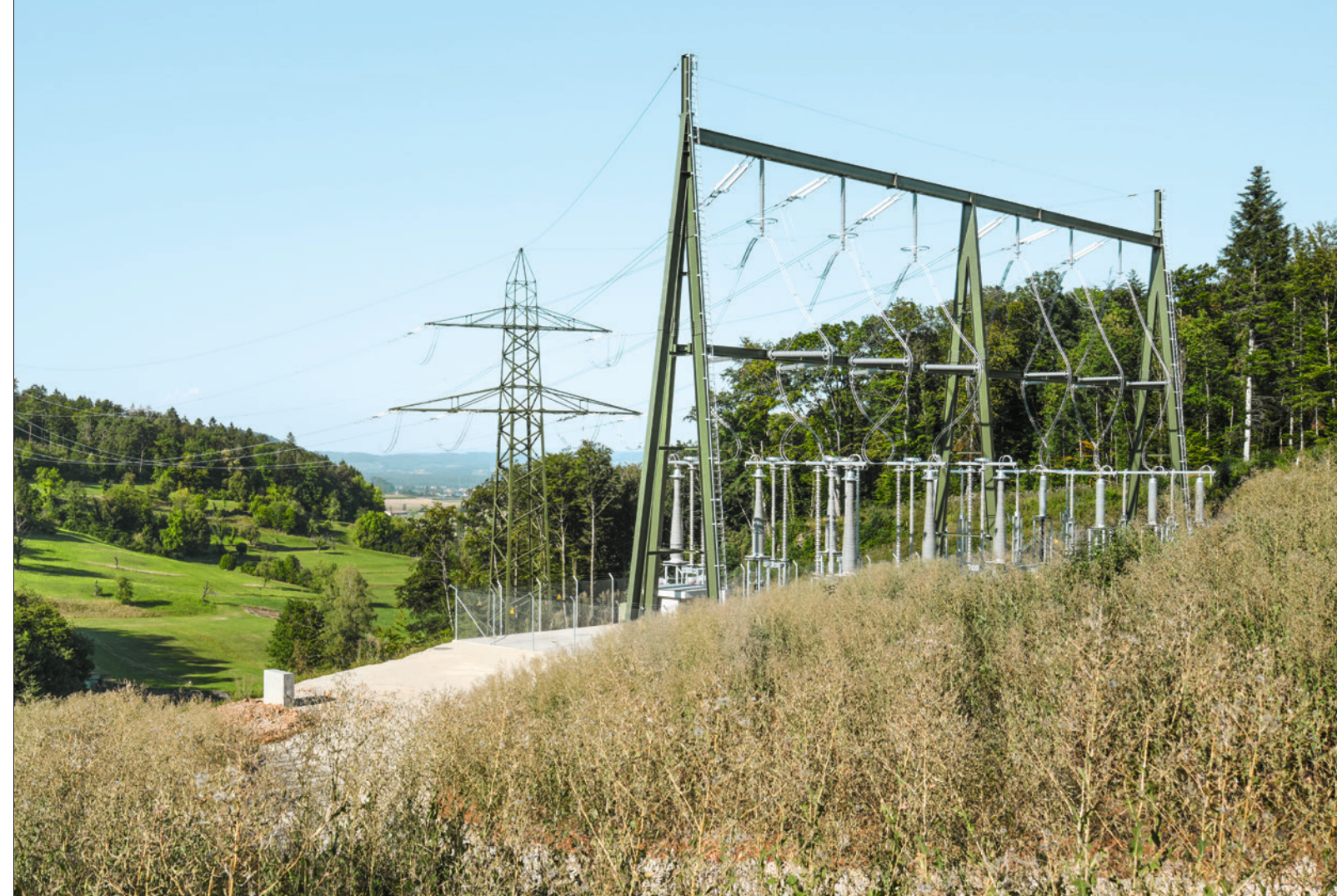
Transitional structure in Riniken (AG) for the Beznau–Birr grid project
